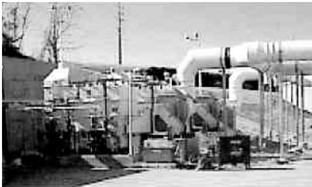
A two-stage chemical scrubber system reduces odor migrating from the Morris Forman facility by removing hydrogen sulfide odor. Combined with the covers on the bioroughing towers, these odor control features cost $3.3 million.
