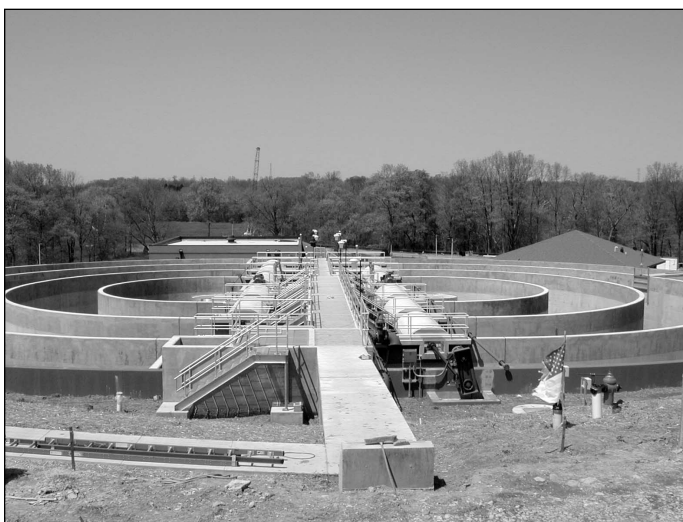
The Floyds Fork Regional Wastewater Treatment Facility (shown here under construction in August 2000) was built with the intent of replacing 11 existing neighborhood wastewater plants in eastern Jefferson County. The Floyds Fork facility began treating wastewater earlier this month.
