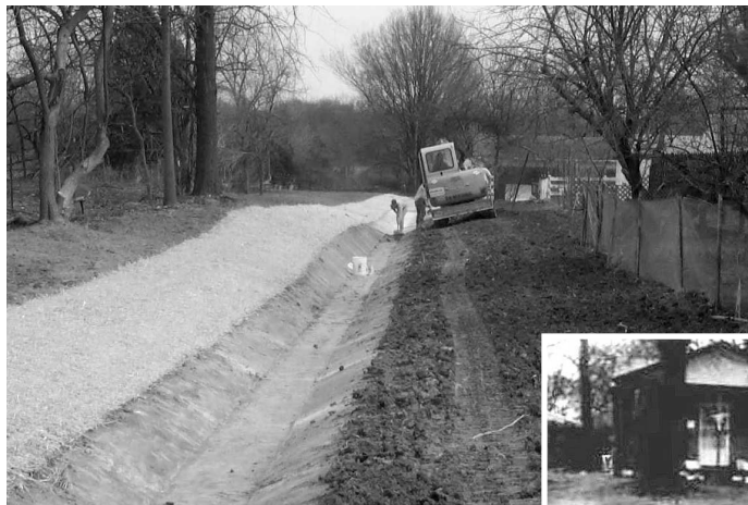
MSD and FMSM Engineers designed a combined system of grass swales and pipe to prevent roadside standing water.
