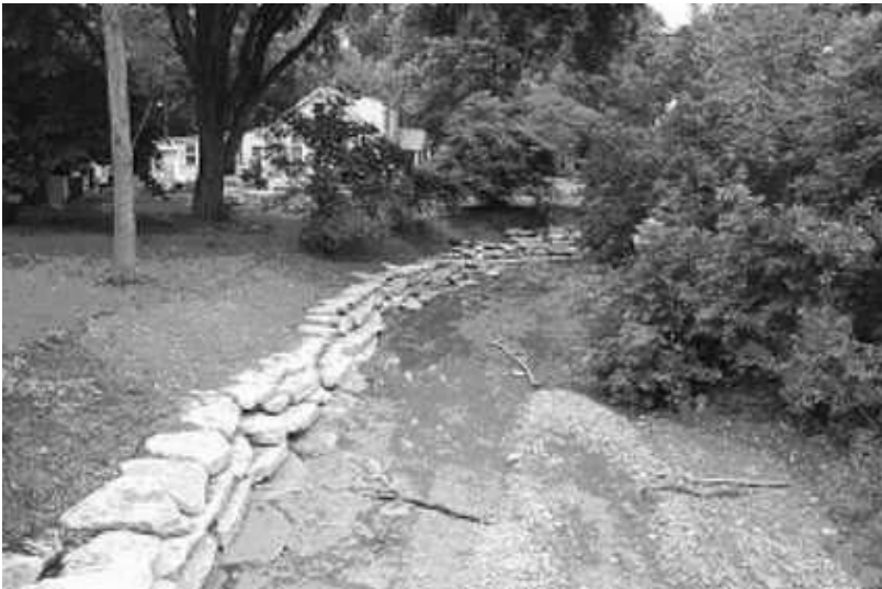
To reduce flooding and improve drainage along Fairdale's Mount Holly Road, a stretch of Little Bee Creek was restored to a more natural state. Other benefits include native bank vegetation and enhanced habitat for wildlife and aquatic life.
