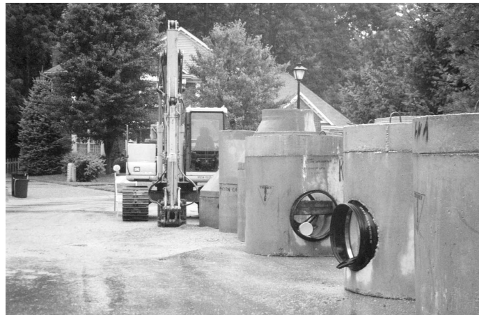
The U of L Center for Infrastructure Research will initially focus on issues for Louisville Water Co. and MSD, who own a combined 10,000 miles of pipe in Jefferson County.
