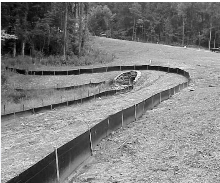
A silt fence keeps construction site sediment from being swept into nearby streams, protecting water quality and reducing the potential for flooding.
