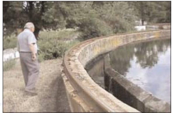
Because investments aren't keeping pace with infrastructure needs, most facilities show signs of significant deterioration.
