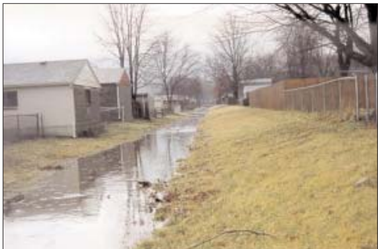
Improvements to this drainage channel will reduce standing water and rear yard flooding between Moody and Blue Lick roads.
