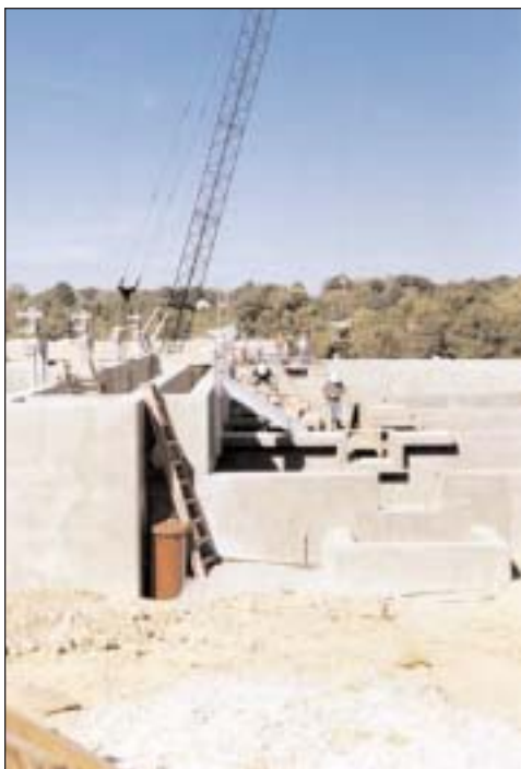
Construction continues to nearly triple the treatment capacity of the Cedar Creek plant.
