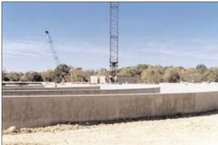
Crews from Cynthiana-based Judy Construction Co. are expanding MSD's Cedar Creek plant. Through the design-build process, other upgrades are being made to enhance plant efficiency and safety.
