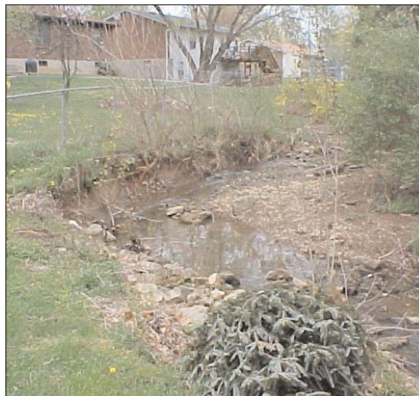
Preventing future erosion along a drainage channel in the Pleasant View subdivision also will reduce private property damage.
