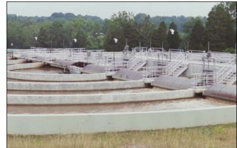
Capacity at Cedar Creek Wastewater Treatment Plant has tripled to serve one of the community's most rapidly growing sectors.
