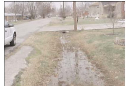
Properties along Tuesday Way will be the first to experience drainage relief as Project D.R.I. gets underway.
