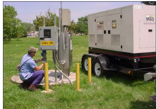
West Region Maintenance Electrician Steve Robbins tests a recently installed junction box on Jacks Lane.
