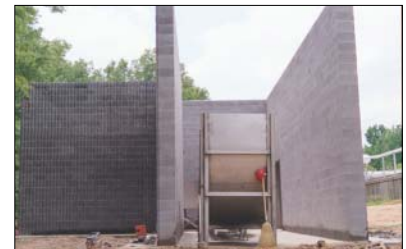
Addition of noise control features on the biofilter blower is underway at the West County plant.
