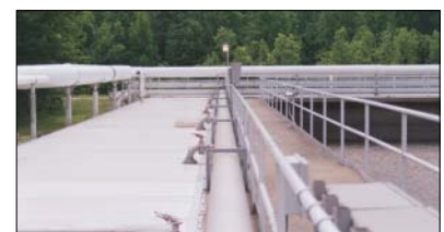
Ductwork moves odor from covered channels to a biofilter. In aeration basins (right) fine bubble diffusers have been installed to help reduce odors.
