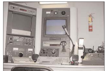
The teleinspection camera sends images from inside sewers to a monitor inside the van, allowing operators to pinpoint the location of blockages in the lines.
