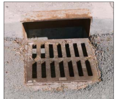
Clogged catch basins can cause localized flooding during heavy rains.
