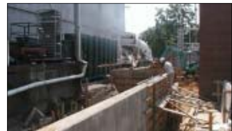
Clearing debris from the Northeastern sanitary trunk sewer will help the renovated Buchanan Street Pump Station operate more efficiently.
