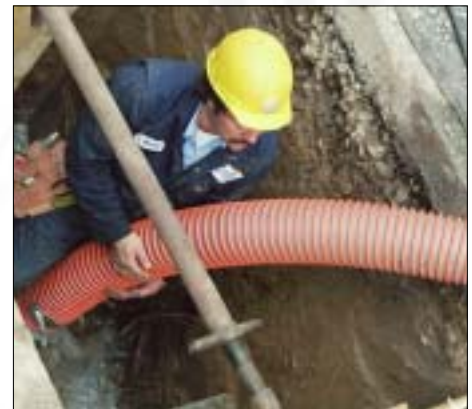
Greg Meredith prepares to repair a sewer line using the new lining system. The new system could save MSD up to 60 percent in costs when used to repair property service connections.
