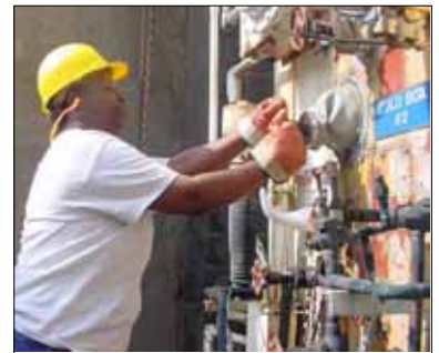
Operator Claudette Thompson adjusts a cold box valve. Upgrades to the oxygen generation area at the Morris Forman plant have increased oxygen production by 35 percent.
