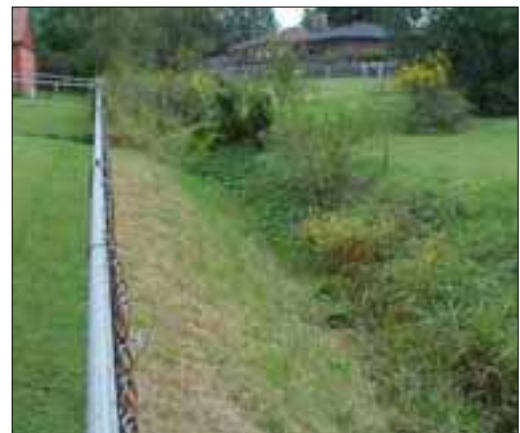
Improving existing drainage systems, like this one in the Pond Creek Area, is part of the Project DRI partnership between Louisville Metro and MSD.
