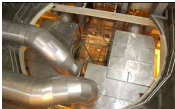
MSD's solids processing system yields about 80 tons of biosolid pellets every day. An employee's idea to keep the tiny pellets from building up in the heat drying system has cut the cost of cleaning them out.
