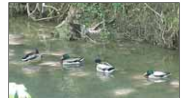
Some Project DRI work includes restoring and stabilizing eroded stream banks. That both promotes drainage and improves stream water quality.
