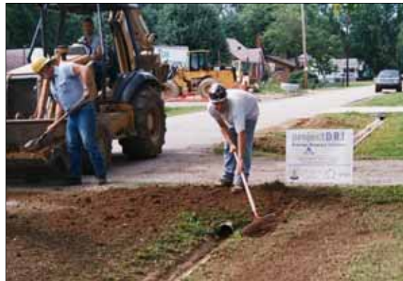
Since Project DRI began in January 2003, drainage facilities have been enhanced or constructed from scratch in neighborhoods throughout Louisville Metro.
