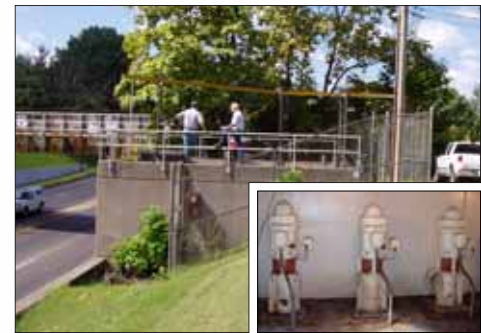
Upgrades planned for two wastewater pumping stations on Algonquin Parkway (above) and 4th Street include replacing pumps that have been in use since the 1920s.
