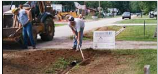
Much of Project DRI work is constructing facilities in neighborhoods that don't have them and upgrading systems that are inadequate.
