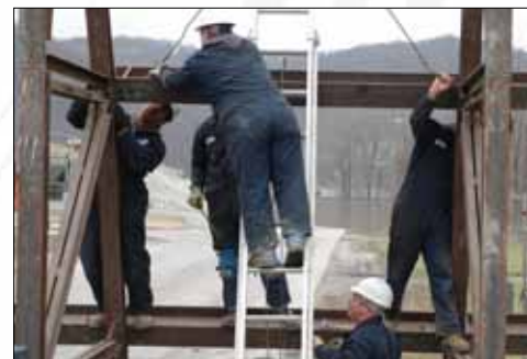
MSD crews installed a street closure as the Ohio River neared flood stage in January.
