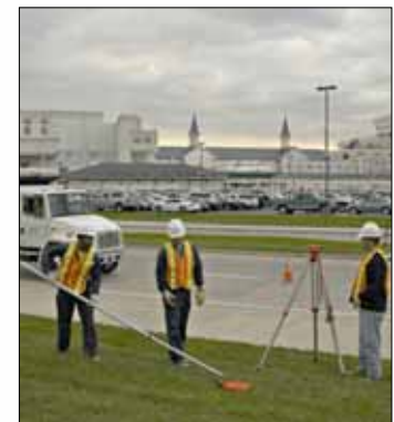
Enoch Dean, David Floyd and Rick Bledsoe check the elevations of a drainage system along Central Avenue.
