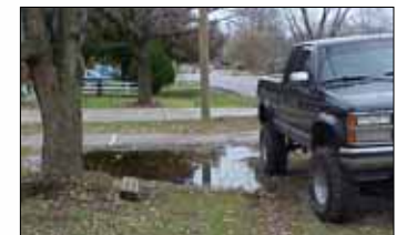
Project DRI will improve roadside drainage along Foreman Lane in Woodland Manor.
