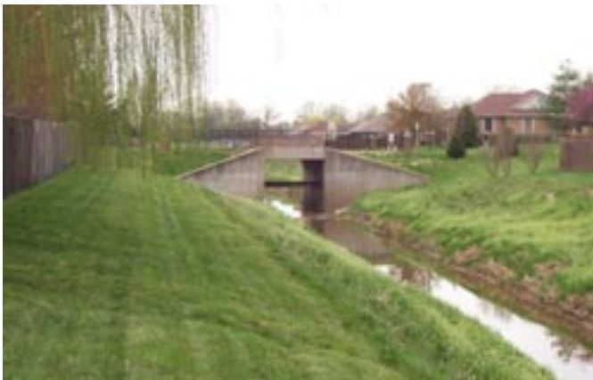
A drainage channel near Lower Hunters Trace is mowed several times a year.
