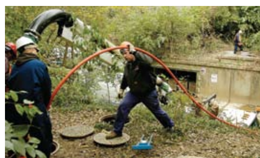
At the present time, crews must access the siphon-outlet manholes by entering the paved channel of Beargrass Creek.
