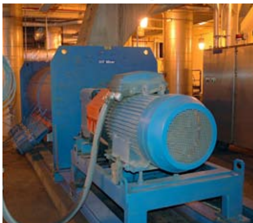
Machinery used to process solids, such as this mixer, are housed in the Main Equipment Building at Morris Forman Wastewater Treatment Plant.
